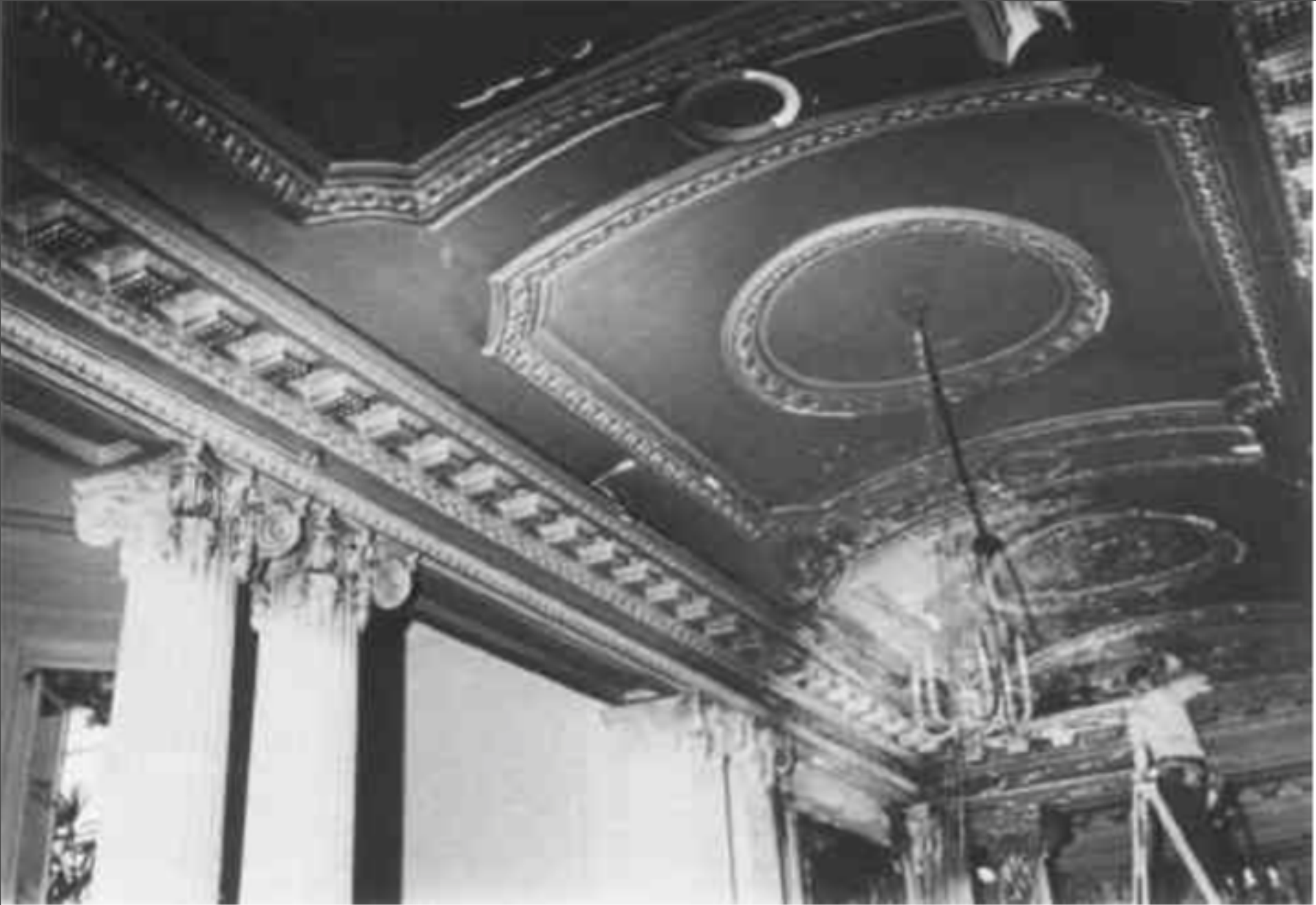
Fig. 1. Huntington Art Gallery—Smoke and heat damage to ceiling in hallway immediately outside elevator shaft.
